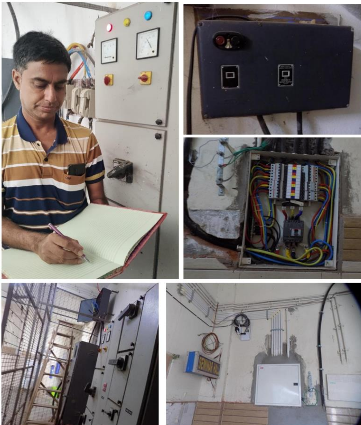
Plate 7. Top left: Energy Audit data collection by Dr. Ayan Bandopadhyay, HOD, Dept of Chemistry, GGDC Chapra; Top-Right & Below-left: Power supply switches and Source room ; Below-right: Newly installed and set up of EI work during Feb 2024 by the PWD te Nadia Electrical Division, Krishnagar, Nadia.
