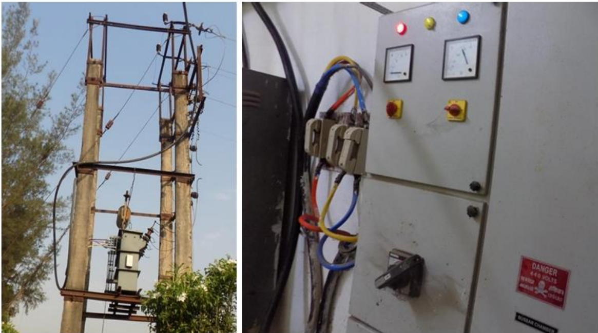
Plate 6. Power Supply with proper safety Guidelines at Govt General Degree College Chapra
