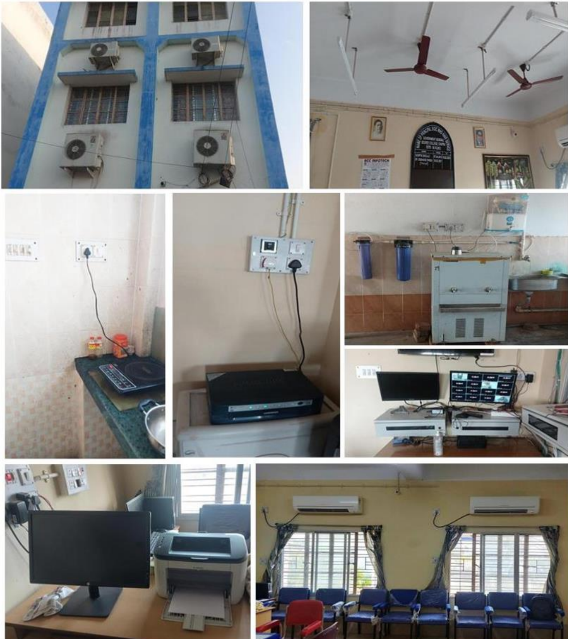
Plate 9. 1 st Row left: AC Block Principal Room & Guest Room; 1 st Row Right: Principal Room LED Light & Fan. 2 nd Row left: Energy consumed by Induction Oven at Canteen; 2 nd Row Middle: Inverter at Principal's Room; 2 nd Row-Right: Energy consumed by Ground Floor Water Purifier system & CCTV Camera at Principal Room. 3 rd Row Left: Computer & Printer at Principal Room; 3 rd Row Right: AC at Principal Room.
